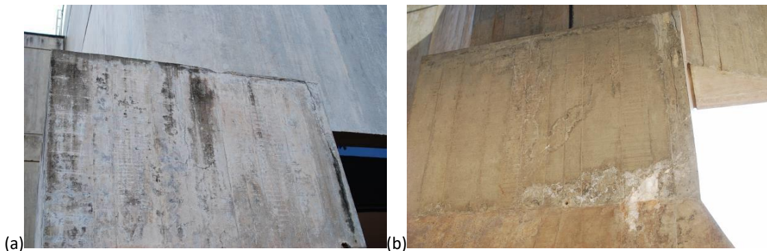
Figure 11 – Superficial spots found in the building – (a) P1B and (b).
