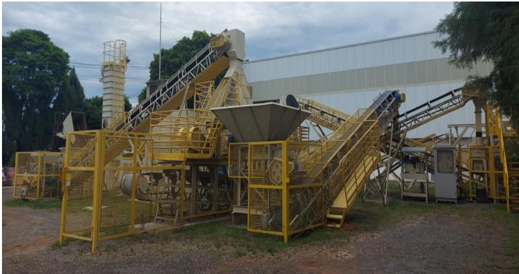
Figure 2 – Overview of the pilot plant used for the tests.
